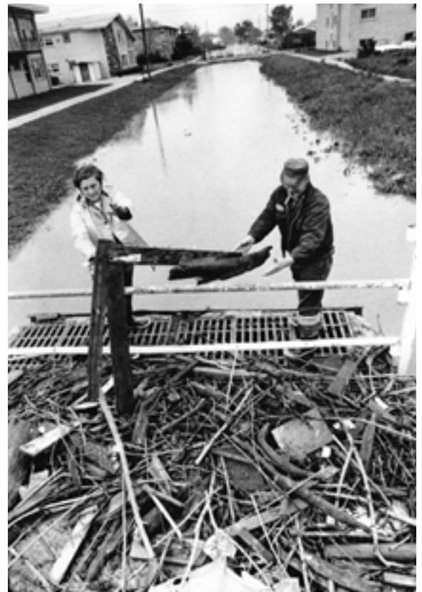
MAY 17, 1974 Don Krueger and Fred Lange clear the Midlothian Creek near 146 th Street after heavy rains caused flooding in the village.
