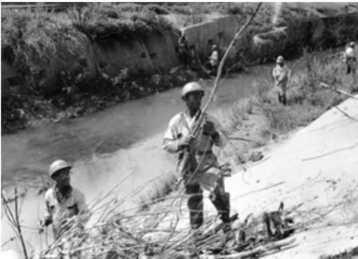
JUNE 5, 1969 Workers clear debris and vegetation from Midlothian Creek at 147 th Street and Hamlin Avenue.
